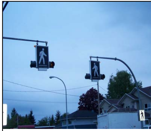
Overhead flashers with beacons
