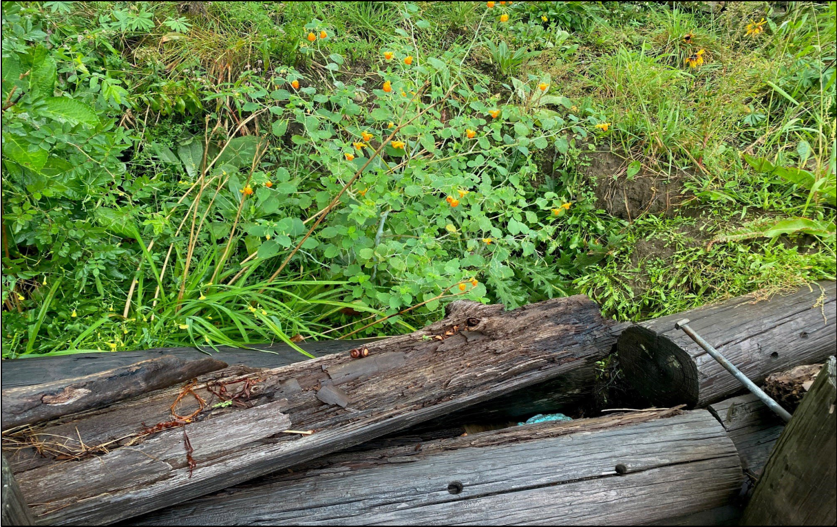
Photograph Five. View of failing timber retaining wall and invasive species.
