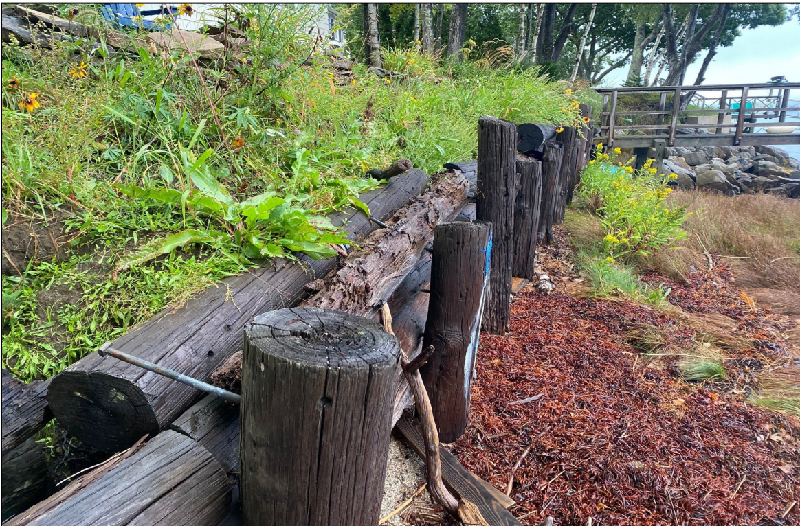
Photograph Four. Existing timber retaining wall on southerly side of dock that will be replaced by riprap.
