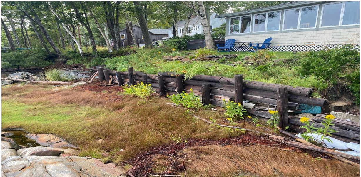
Photograph Eight. View of timber retaining wall and intertidal zone facing northwesterly.
