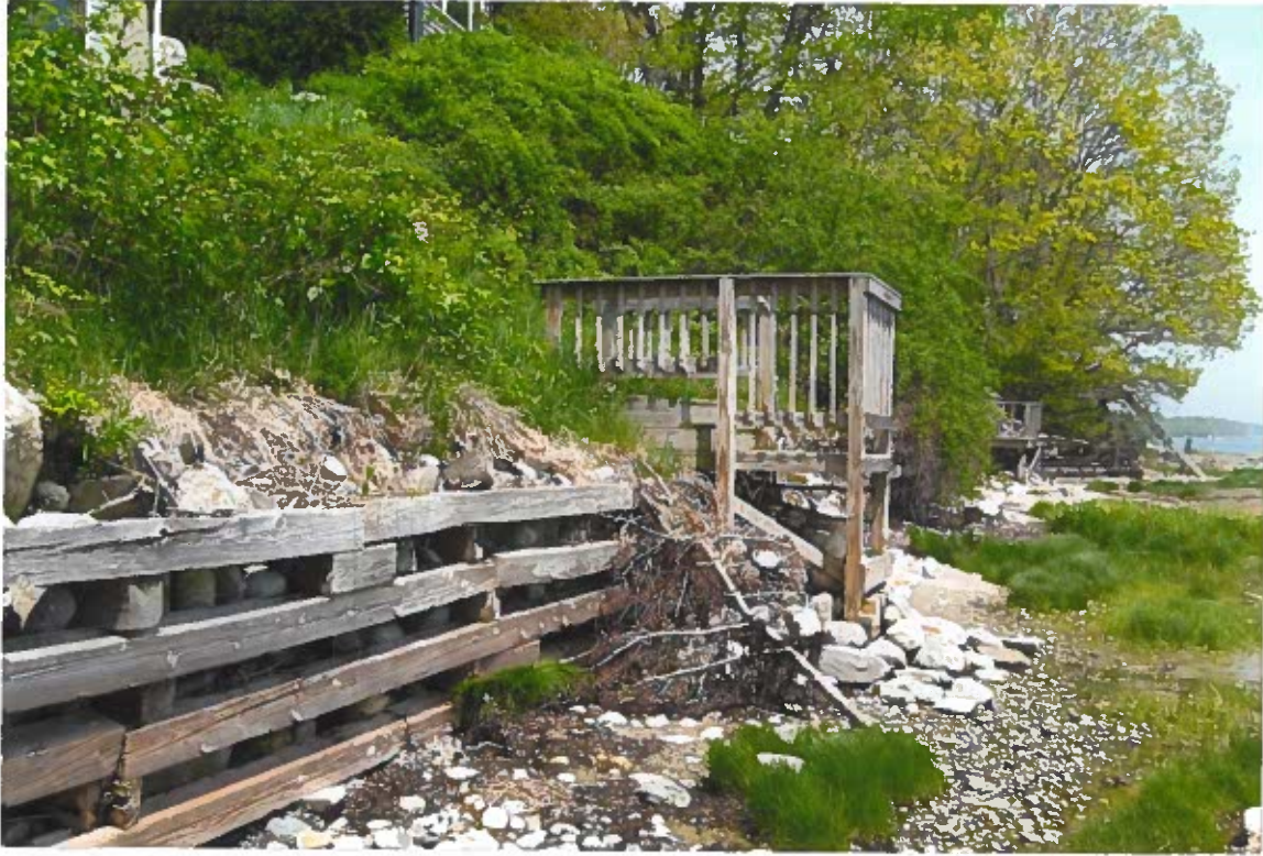
Retaining wall and stairs before 2022 storms
