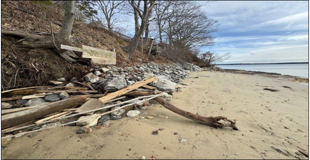
Photograph Three. Additional view facing northeast. Additional view of exposed shoreline where riprap has washed down slope.
