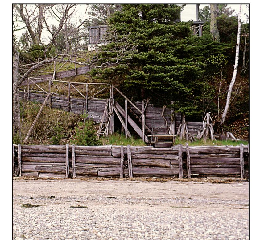
Stable bluff with a vegetated bluff face and an armored shoreline. The bluff face is fully vegetated and supports a mature stand of trees with vertical trunks. The presence of a wooden bulkhead suggests that erosion has occurred in the past.
