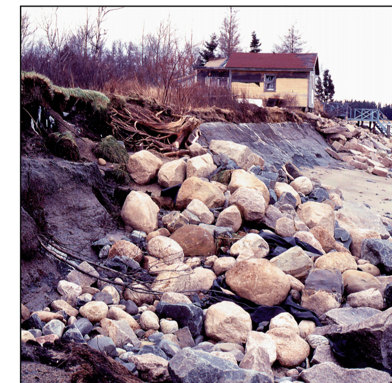
Highly unstable bluff with an unvegetated bluff face and an armored shoreline. This armored bluff is eroding despite an effort to shore it up with riprap, or loosely piled stone blocks. Maintenance at this site could improve bluff stability.
