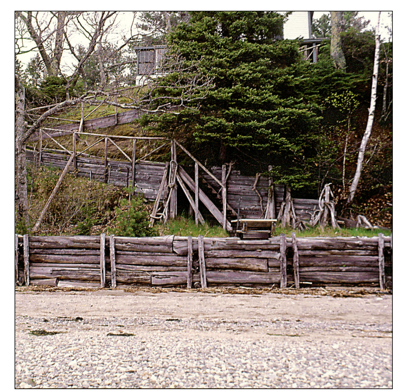
Stable bluff with a vegetated bluff face and an armored shoreline. The bluff face is fully vegetated and supports a mature stand of trees with vertical trunks. The presence of a wooden bulkhead suggests that erosion has occurred in the past.
