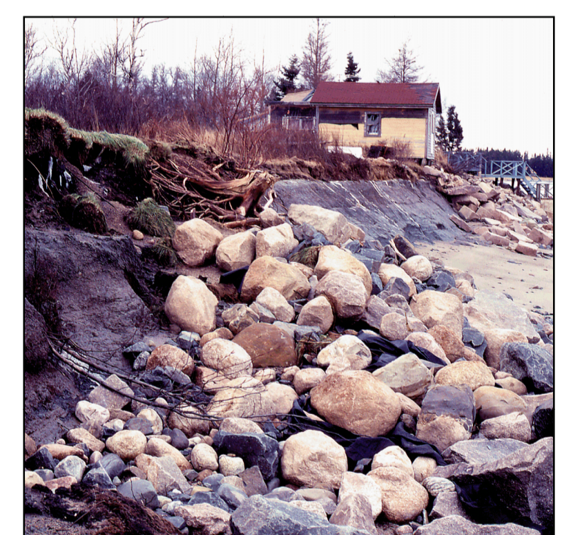
Highly unstable bluff with an unvegetated bluff face and an armored bluff face. This armored bluff is eroding despite an effort to shore it up with riprap, or loosely piled stone blocks. Maintenance at this site could improve bluff stability.
