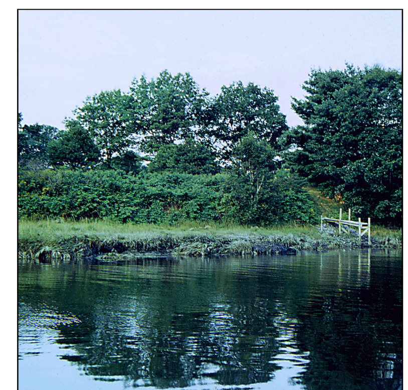
Stable bluff with a vegetated bluff face and a salt marsh shoreline. A low bluff face is covered by shrubs landward of a salt marsh terrace. In this location the nature marsh protects the base of the bluff from rapid erosion and slows bluff recession or retreat.
