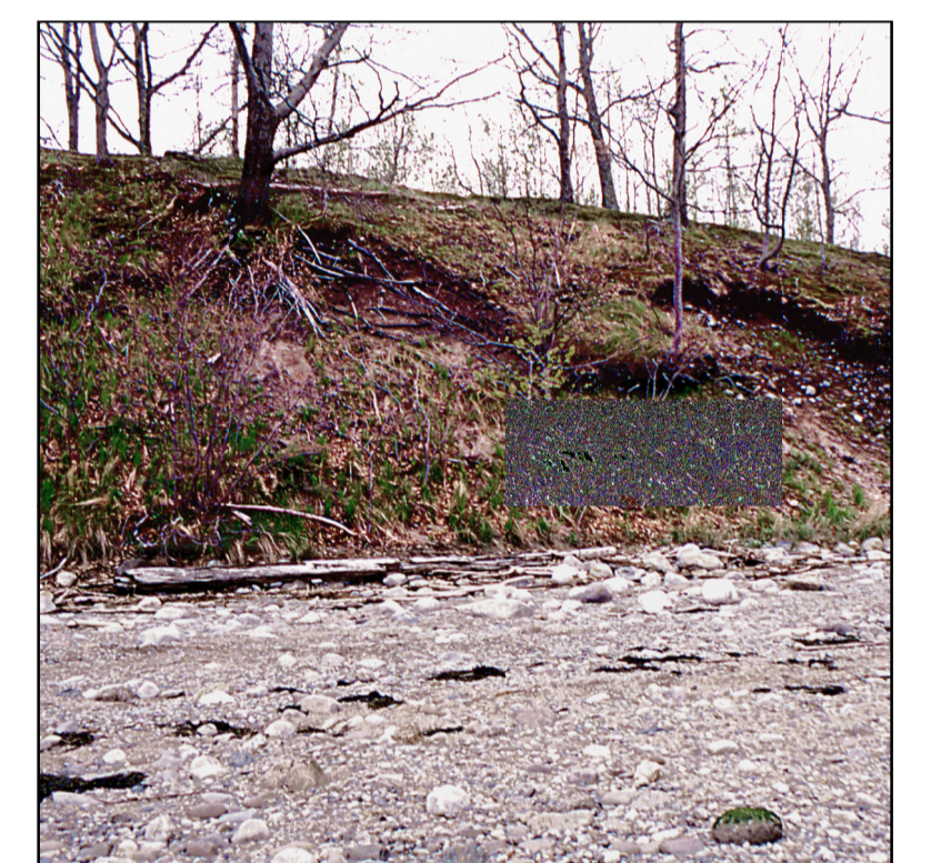
Unstable bluff with a partially vegetated bluff face and a beach/gravel flat shoreline. Slump scars on the bluff face expose sand, gravel, and roots. Fine sediments are removed by waves and currents, leaving gravel to form a beach at the base of the bluff.
