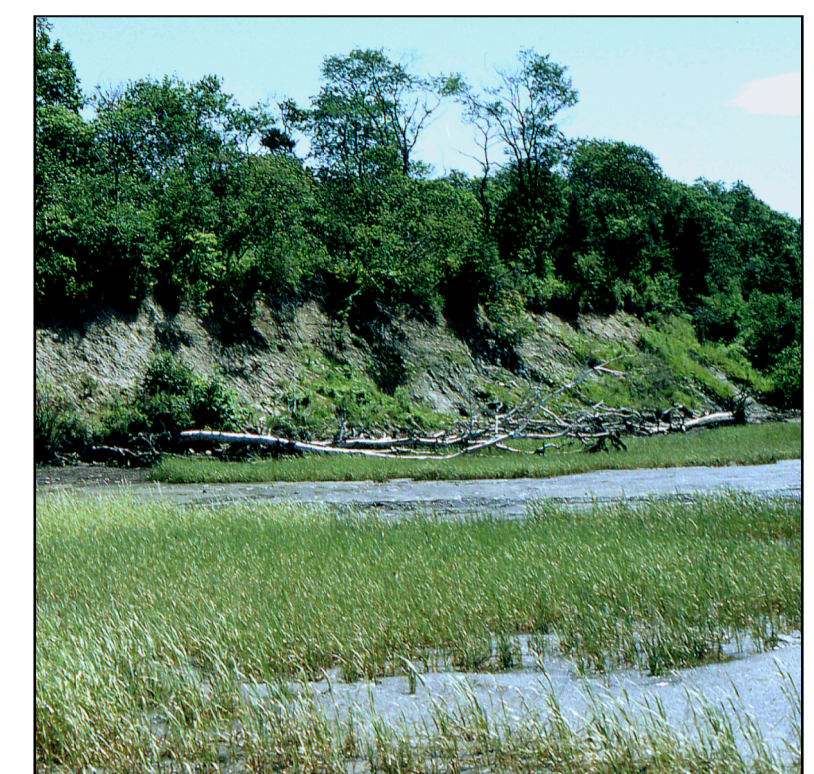
Highly unstable bluff with an unvegetated bluff face and a salt marsh shoreline. Sediments on the bluff face are exposed and fallen tree trunks lie at the base of the bluff. A salt marsh has recently formed on the tidal flat, partly on the top of an old landslide deposit.
