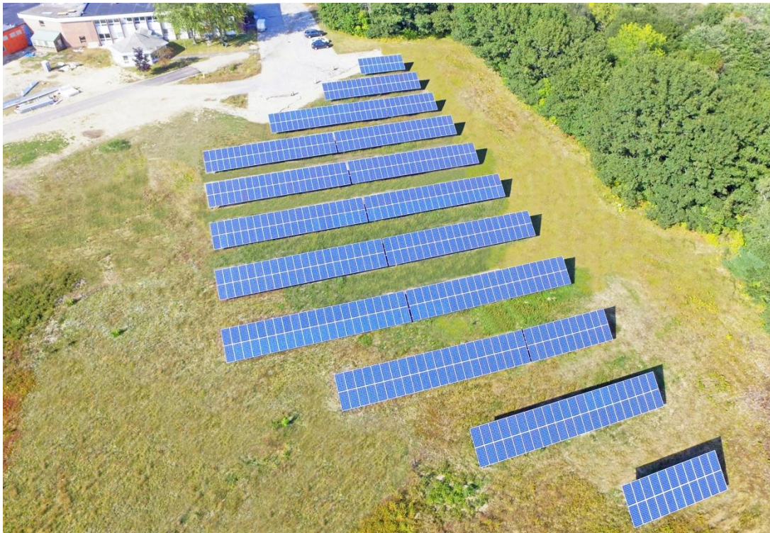
Geiger - Lewiston, ME 233.16 Kilowatts (696 solar panels)
