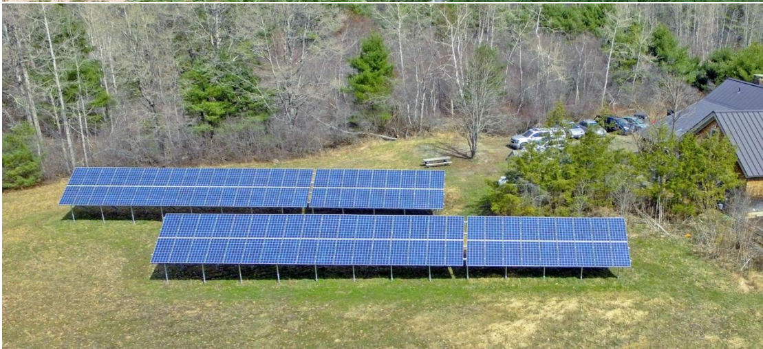
Little River Veterinary Hospital – Northport, ME 27.56 Kilowatts – multiple views
