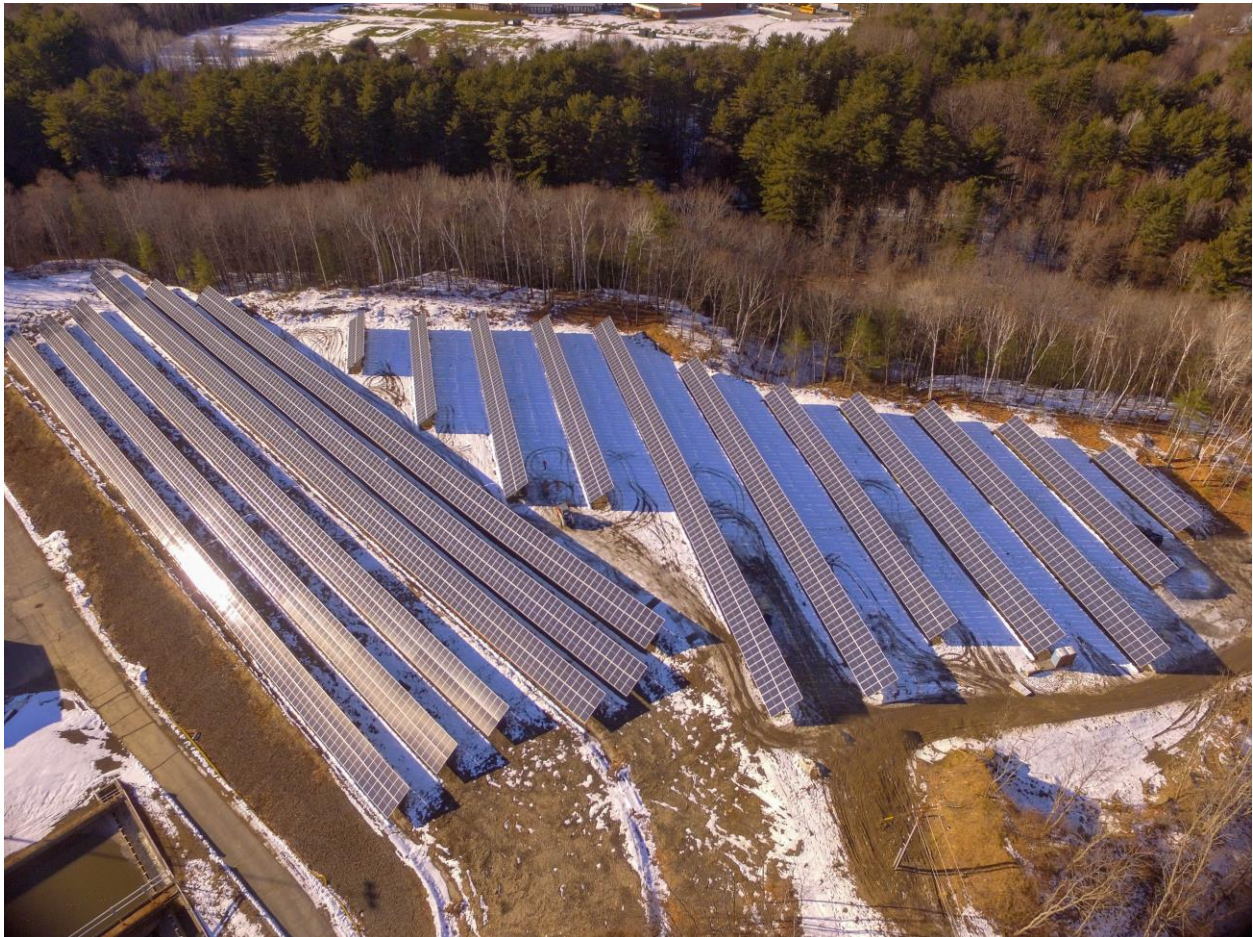
Figure 1. A 968.76 kW solar array installed for the Kennebec Sanitary Treatment District in Waterville, Maine, by ReVision Energy.
