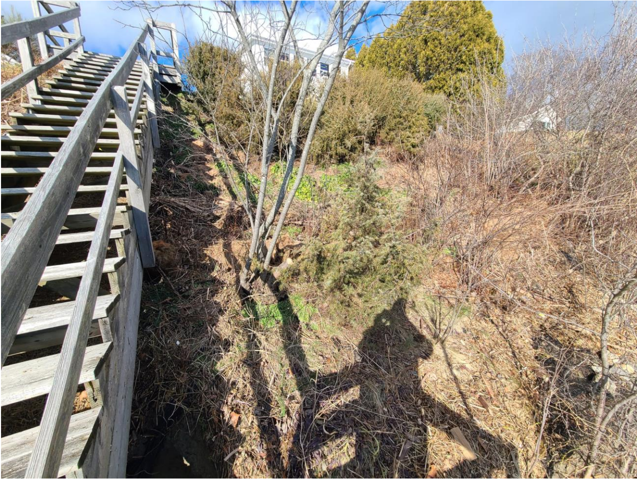
Photograph Three: Facing North West—view of dramatically eroding shoreline with multiple cuts into the embankment and view of the exposed soil and the undercut bank in area of proposed stabilization.
