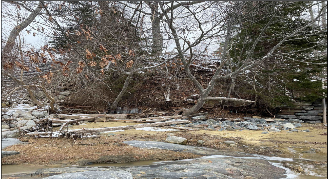
Photograph Two. Proposed area of riprap including existing stone wall and wooden access stairs to the right. One of the trees pictured will need to be removed to install the riprap.
