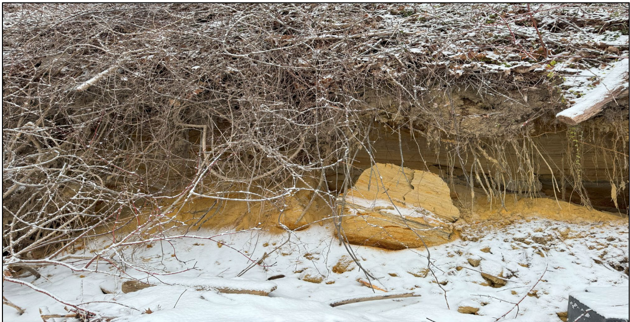
Photograph Two. Portion of base of slope that has been undercut. Woody vegetation will need to be removed to install riprap.
