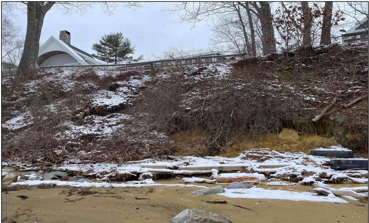
Photograph Five. Additional view of undercut shoreline.
