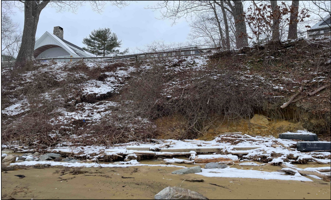
Photograph Five. Additional view of undercut shoreline.
