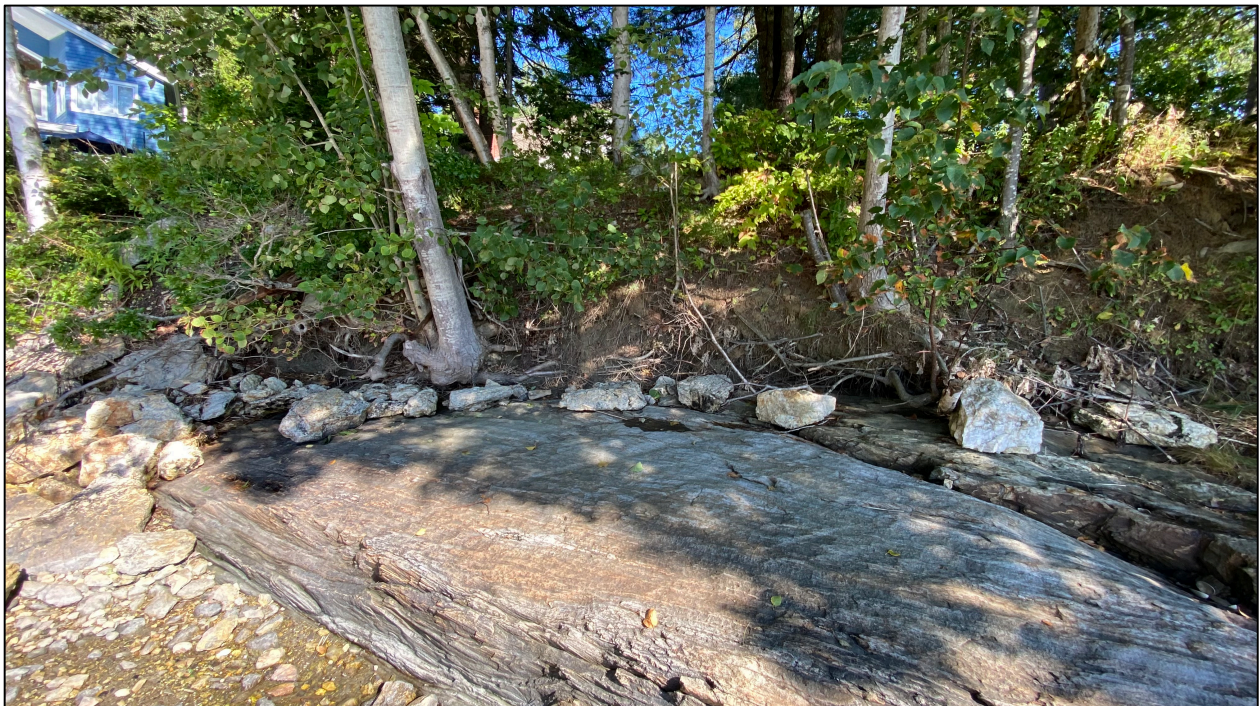
Photograph Six. Additional area of shoreline that is exhibiting erosion that is proposed to be stabilized with riprap. Photographer: Tim Forrester, Atlantic Environmental, LLC. Date: September 8, 2022.
