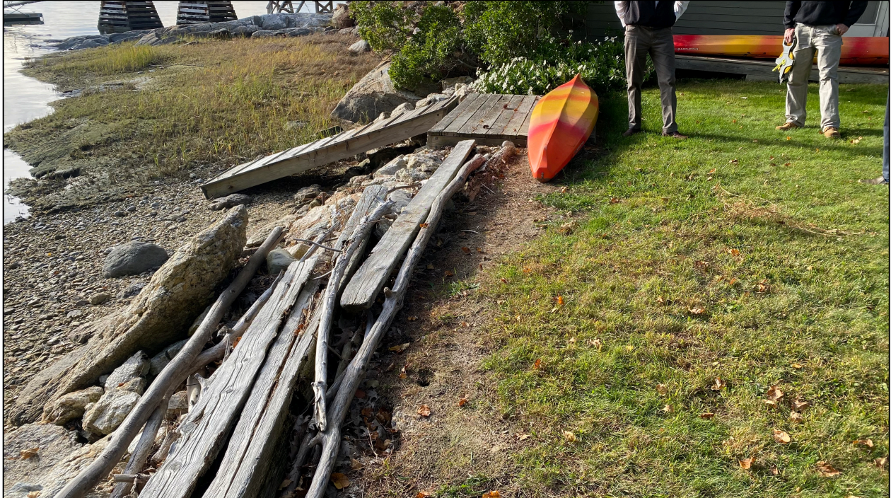
Photograph Five. View of area that is eroding behind existing riprap. Photographer: Tim Forrester, Atlantic Environmental, LLC. Date: October 4, 2022.
