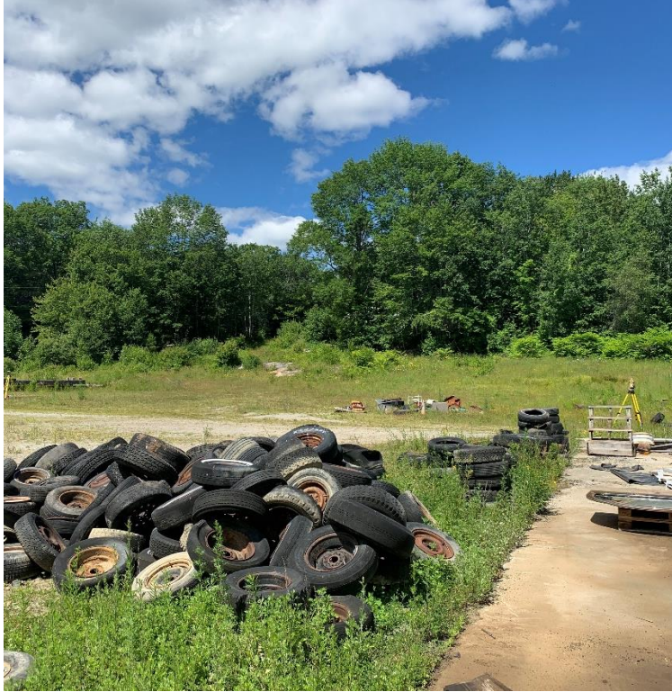
Photo 5. From new building location looking toward western property line (July 2022, debris has been removed)
