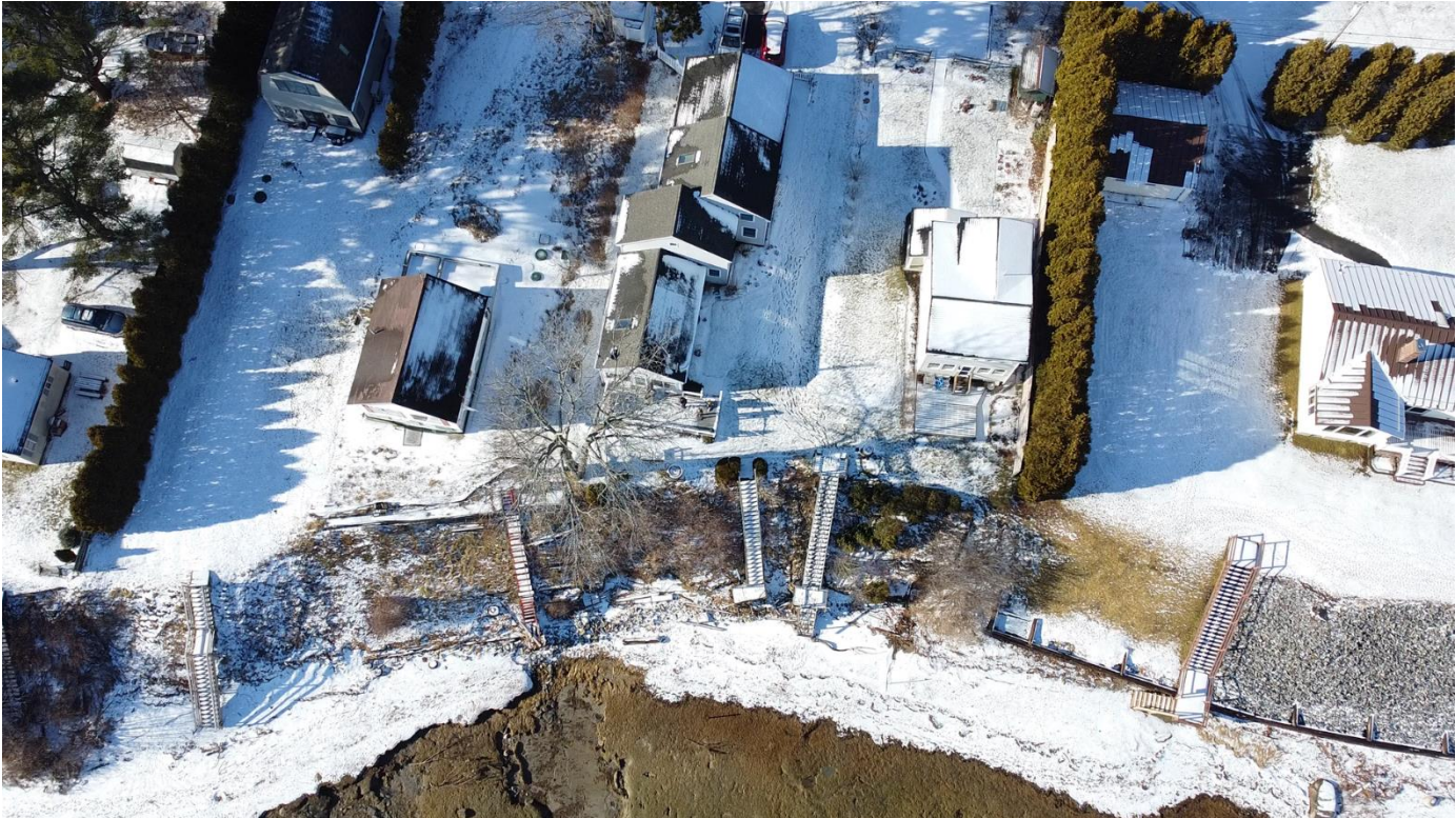
Photograph Four: Drone shot of Eroding shoreline and neighbor riprap to the top of their embankment.
