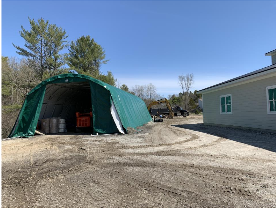
Figure 3. Previous “dome tent”, new tent will be of similar style and color
